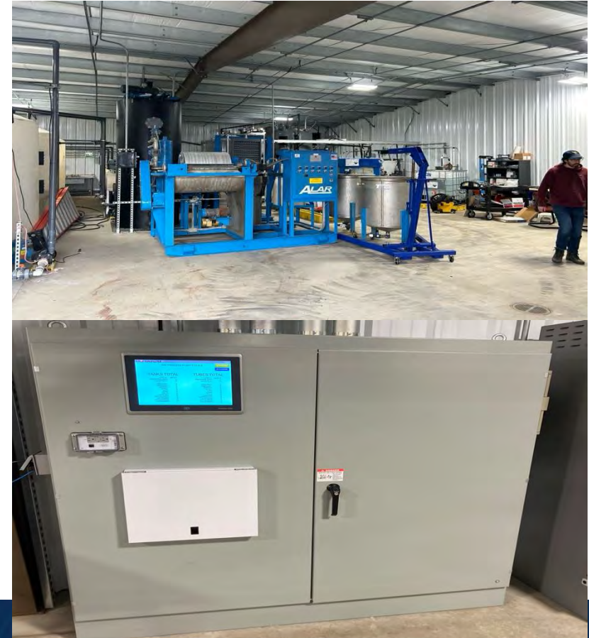
Top: High Solids Leach Circuit, Bot: Automation Cabinet
